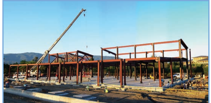
An early photo of the water quality lab under construction showing the steel beams and concrete slab.
